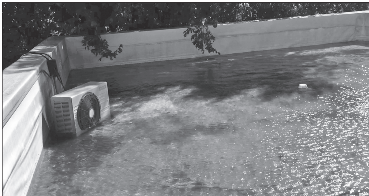
STANDING WATER POOLS on a roof atop the old Green Lake County courthouse. A big elm tree next to the building drops leaves, which clog the drainage system. The beloved tree was poised to be cut down, but its fate has been reconsidered. submitted photo
